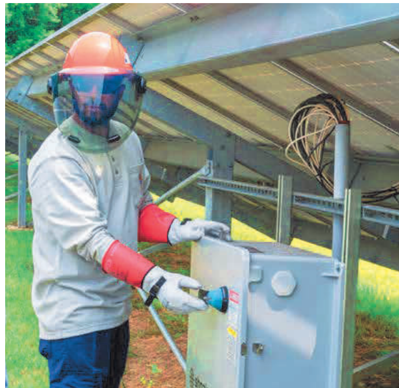
Figure 13-9: When a ground fault is known to be present, technicians should wear appropriate PPE and avoid direct contact with any exposed metal components.
