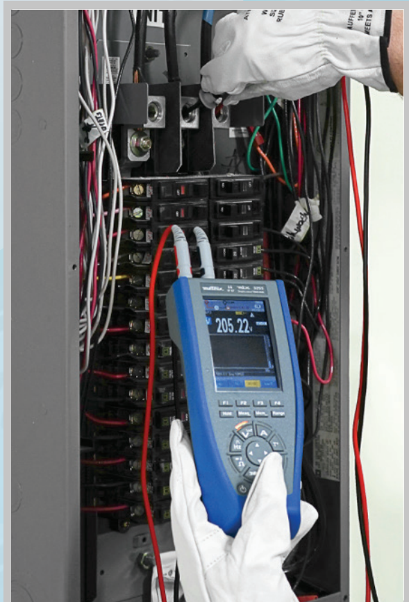
Measurements on electrical cabinets
