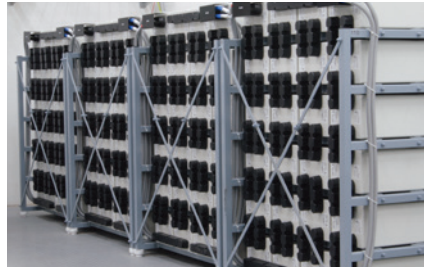
Energy Storage System
